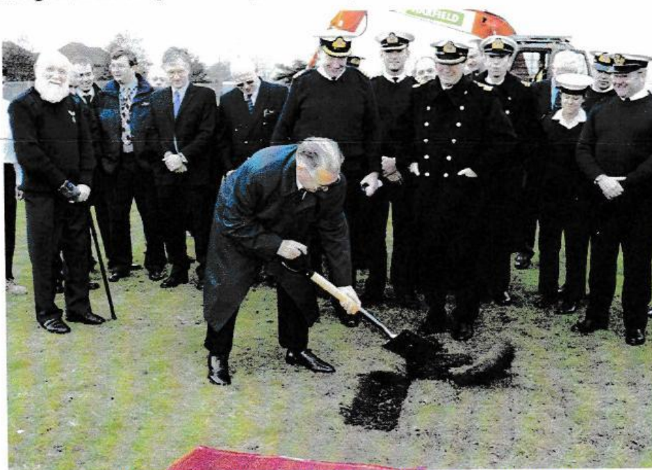
Ted Briggs digging the first turfs to mark the start of construction
